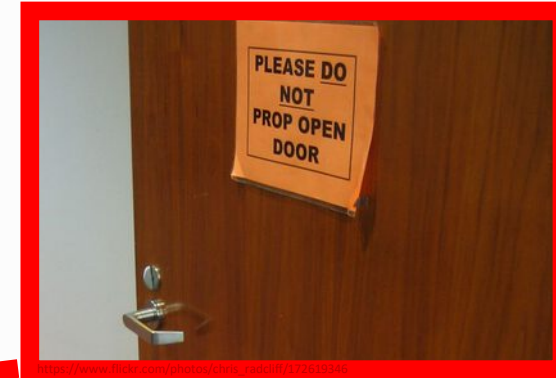
Server Room Door Propped Open
