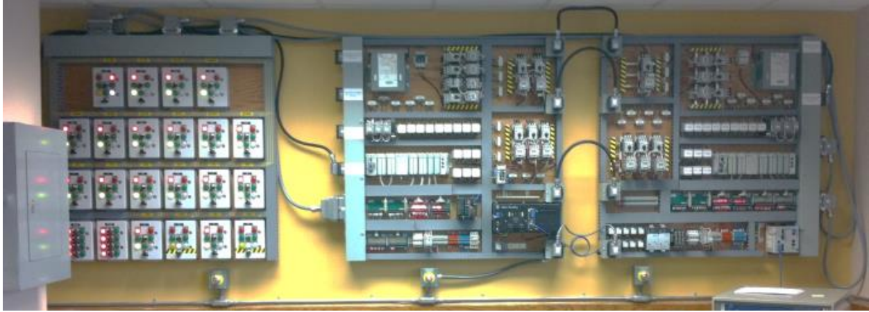
Figure 13 - Ring-type electric power substation testbed located in the Henneke building at the University of Tulsa
